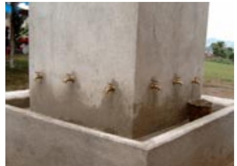
The new school includes this structure for washing hands that has its own water supply.
